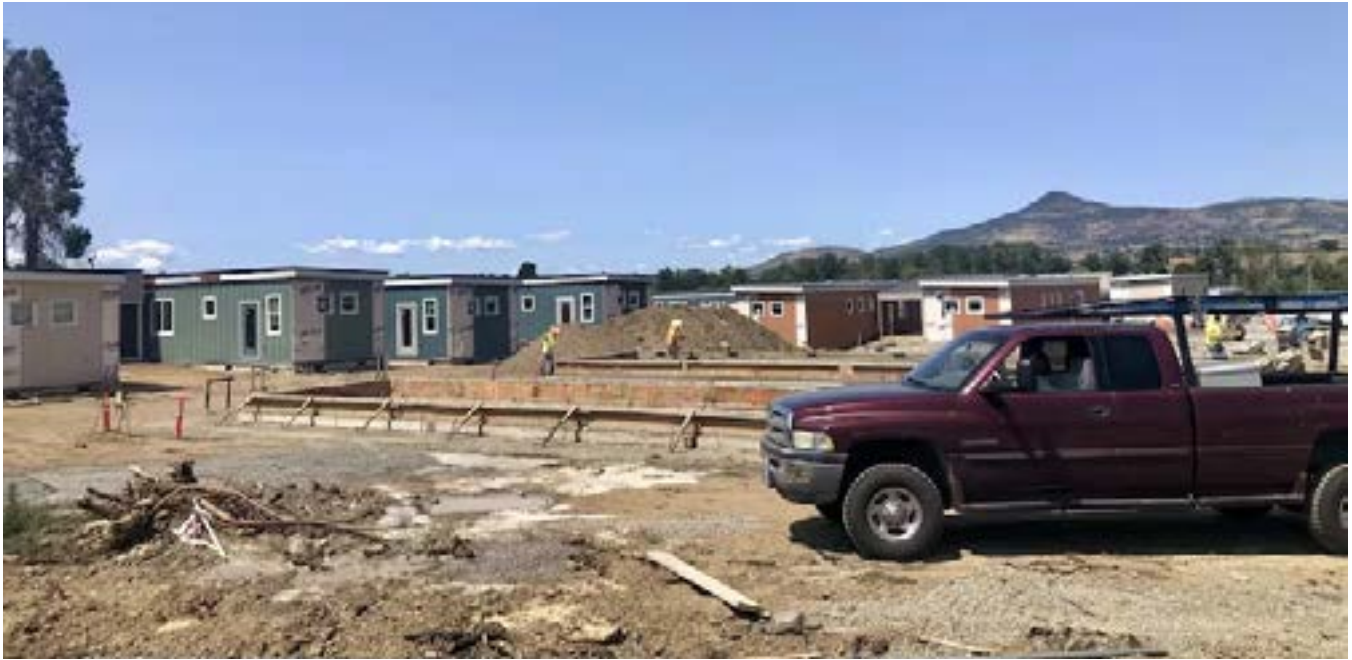
Defective homes marked for removal in Phoenix, Oregon. Source: Jane Vaughan, JPR
